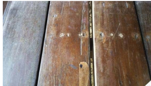
FIGURE 12. Chengal hardwood timber floor (view from inside) with the gaps between each panel.
