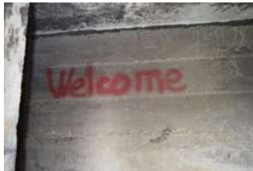
Figure 13: Traces of vandalism on the wall of the entrance of the pillbox at Kg. Anak Rhu, Bachok, Kelantan. Source: Field study.
