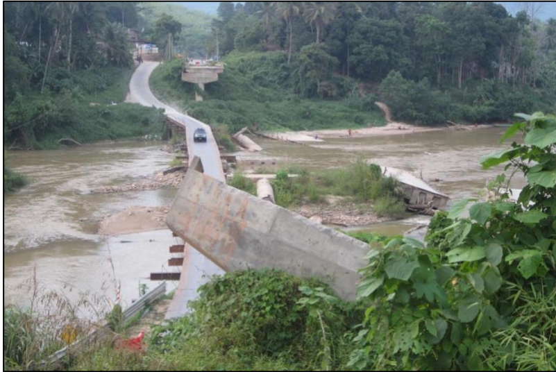
Plate 11: The fury of nature in Stelu, Kelantan, an aftermath of a big flood that hit Peninsular Malaysia's east coast in 2004. A makeshift bridge was constructed and used next to the collapsed bridge.
