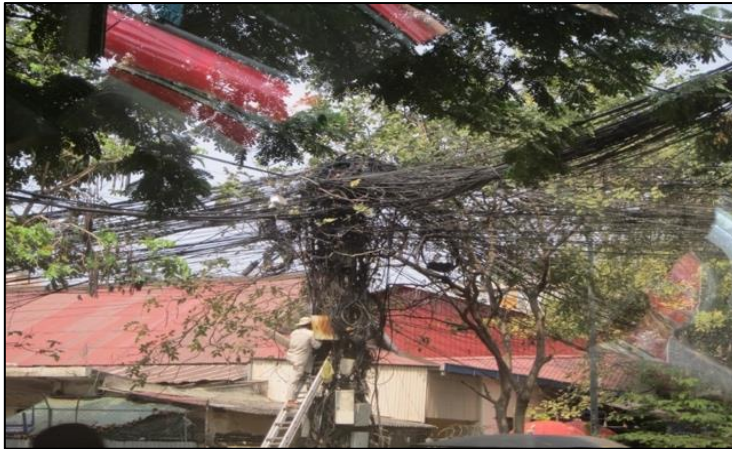
Plate 6: A massive web of communication and electrical lines in Phnom Penh, a relatively common sight in less developing countries.
