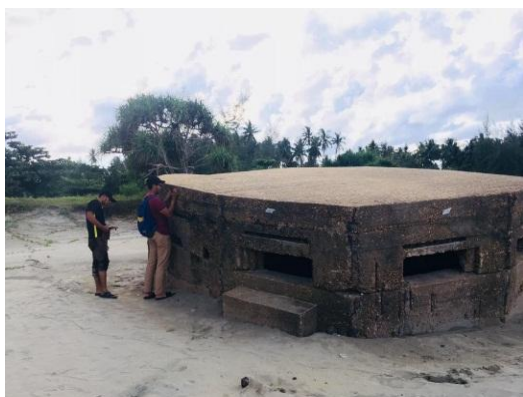
Figure 10. Observation of damage to pillboxes
