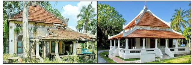
Figure 3. Picture shows before and after the component damage of the building due to plant invasion in Kg. Gadong mosque, Rembau Negeri Sembilan. (Source: website ntqt.com.my)
