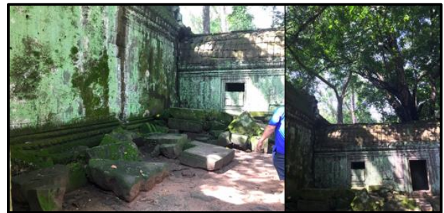
Figure 1. Dampness level on the walls of Ta Prohm temple, Cambodia causing moss and green stains due to plant or tree canopy blocking the sunlight from reaching the lower part.
